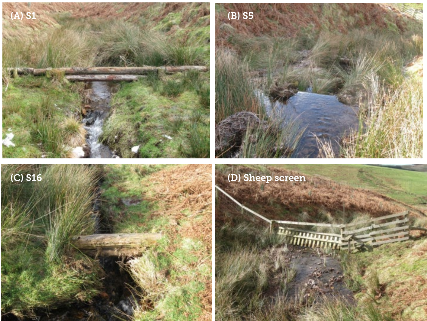
Figure 40: Selected range of geomorphic responses observed during the February 2016 survey (following several high flows in December 2015 and January 2016). Refer to Figure 38 for the locations of these sites. (A) Vertical scour of up to 0.35 m below a flow restrictor. (B) Deposition of 0.85 m 3 of material upstream of a flow restrictor (C) Scour of up to 0.1 m underneath a flow restrictor and trapping of debris. (D) Deposition of 2.9 m 3 of sediment upstream of the sheep screen at the upper end of the fenced enclosure.
